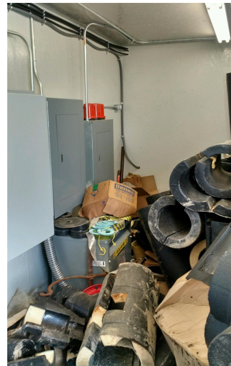
An excellent example of completely inadequate working space around equipment.
